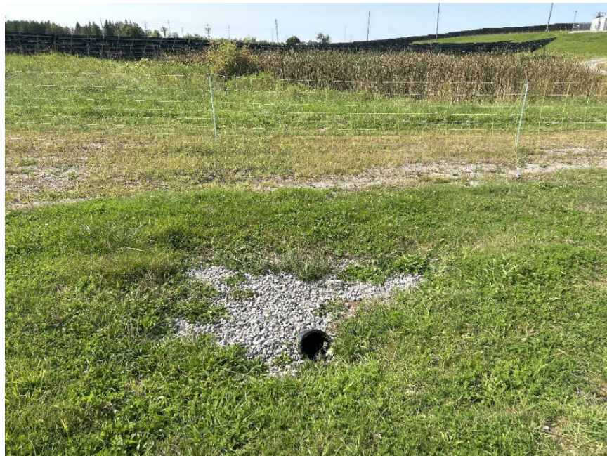
Photo 2 Culvert under access laneway conveying ephemeral drainage between wetland pockets at headwaters of mapped watercourse on the Site, September 2023.
